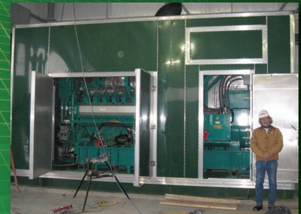
A 1.1 MW Genset at our 3.6 MW Utica, NY CHP site
